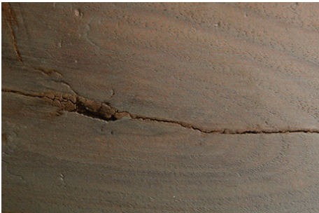
Kleine Risse Cracks in wood
